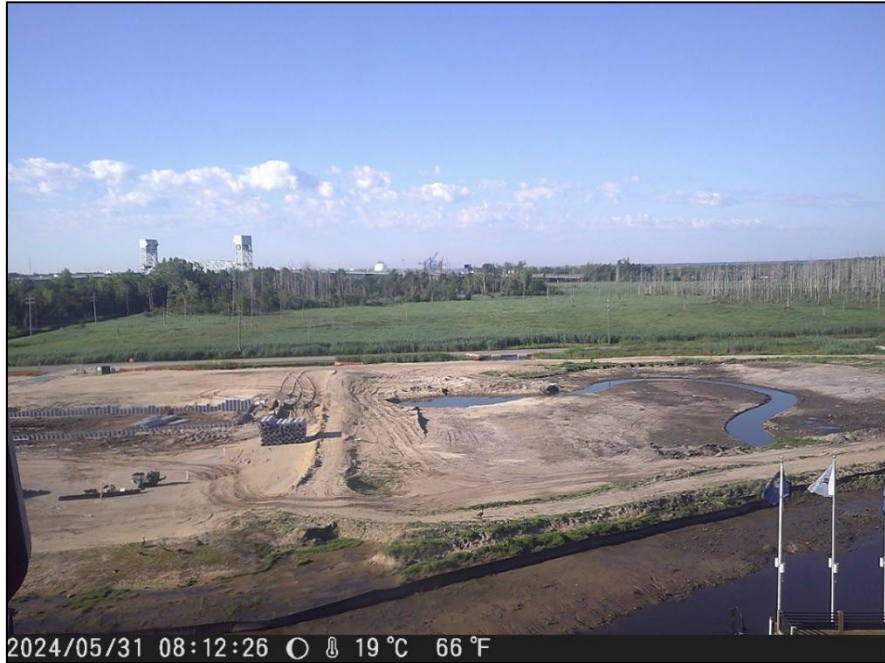
Appendix B-5. Construction camera on the south (port) side of the USSNC on May 31 st , 2024.
