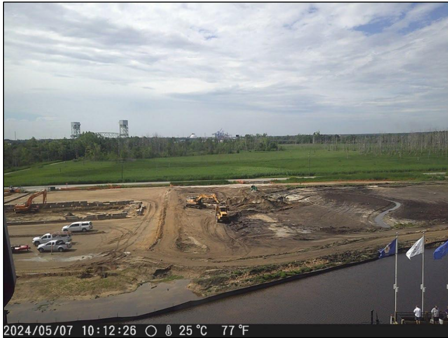
Appendix B-1. Construction camera on the south (port) side of the USSNC on May 7 th , 2024.
