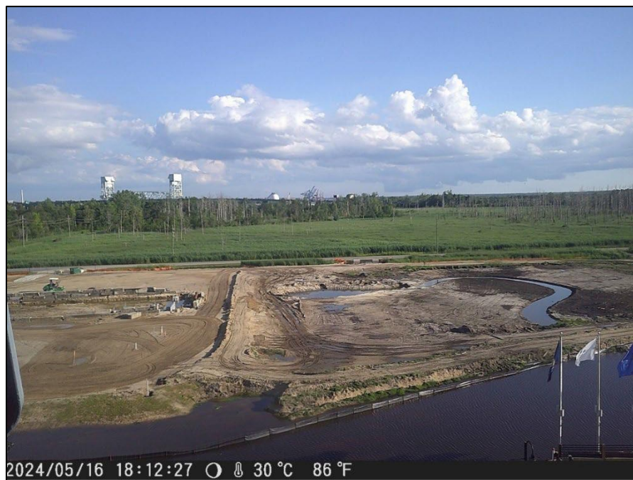
Appendix B-2. Construction camera on the south (port) side of the USSNC on May 16 th , 2024.
