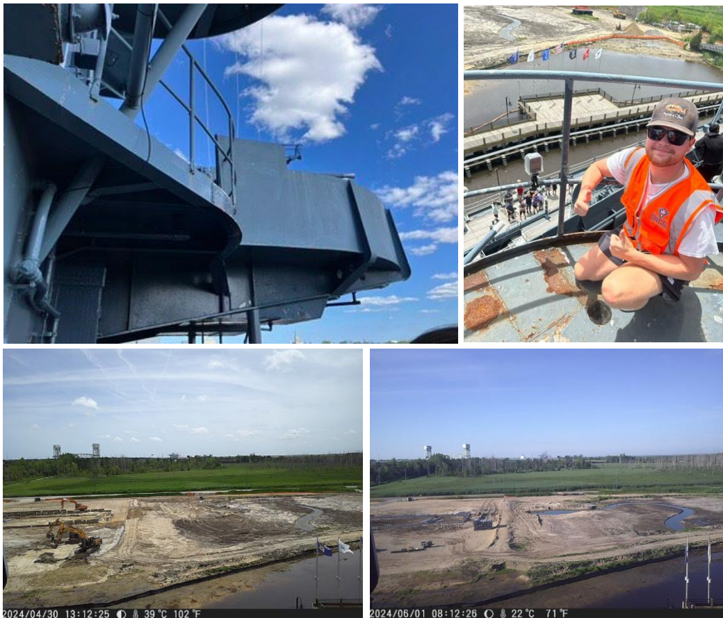
Figure 18. Construction camera on the south (port) side of the USSNC (top row) to capture progress on the constructed wetland, such as changes in the local hydrology due to the newly constructed tidal creek (bottom row). See Appendix B-1 through B-5 for more imagery.
