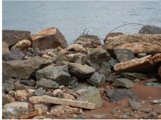
096 - Concrete rubble and rebar in revetment near Location 11.
