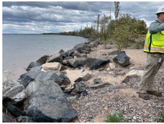
159 - Newer revetment extension at Hawley Street intersection, geotextile is exposed. Location 17.
