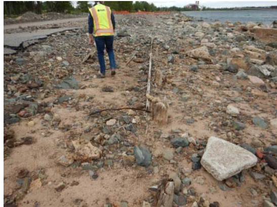
105 - Exposed timber pile bulkhead with tie-back remnants, near Location 11.
