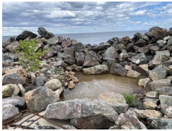
061 - Successful ad-hoc protection of stormwater outfall. Location 6.
