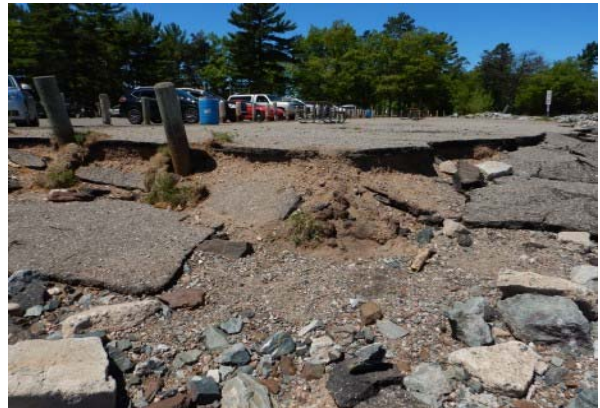
008 - Eroding shoreline and colapsing asphalt from the parking lot at Shiras Park. Location 1.
