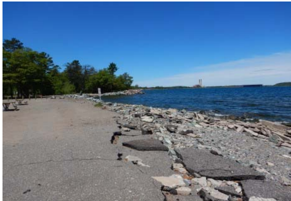
014 - Looking north along the shoreline from Shiras Pake Not ad-hoc armoring and colapsing asphalt. Location 1.
