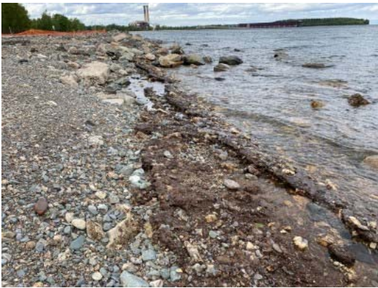
097 - Exposed iron-slag-cobble conglomerate along the project shoreline. Between Locations 11 and 12.
