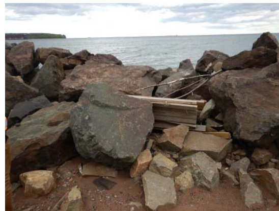
134 - Woody debris in revetment near Location 13.
