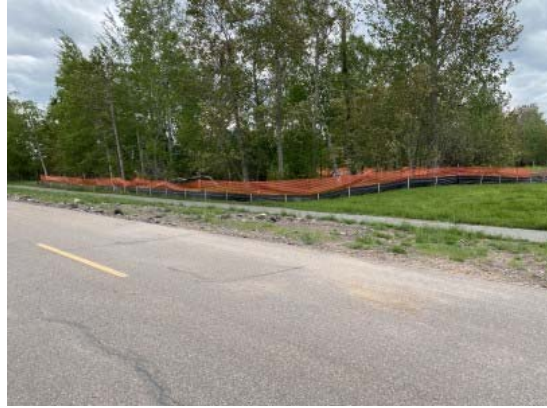
145 - Largest piece of existing wetland on project site, fenced off during roadway construction. Near Location 14.
