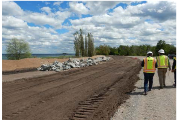
014 - Armor purchased by the city for temporary protection of the roadway. Location 4.
